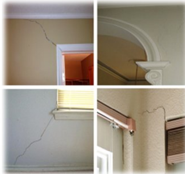
Fig.1: Cracks that appear in walls around architectural openings like doors and windows over time.[3],[4],[5],[6]
